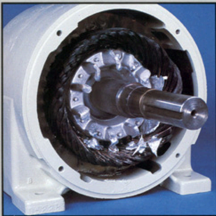
11 Damage Caused by Locked Rotor
